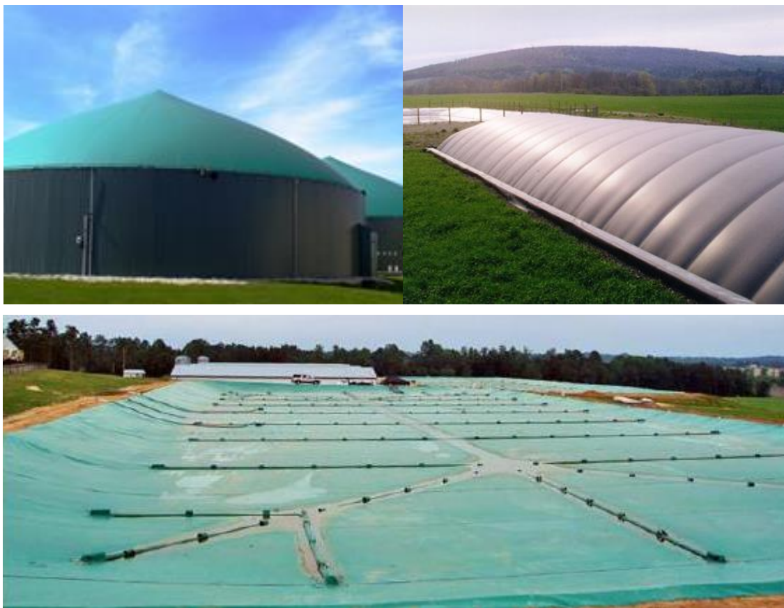
Figure 32: Complete-mix tank (top left), plug flow (top right), and complete-mix lagoon (bottom) anaerobic digesters.
